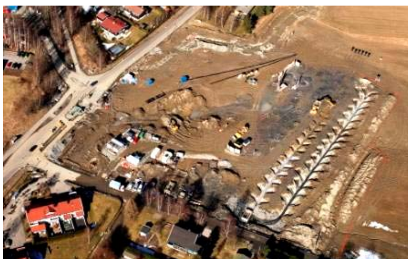
Figure 10: Overview of the 20,000 m 2 area for the thermal energy storage (Ahus, 2008).
