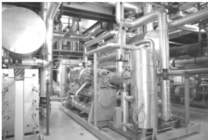
Figure 9: Ammonia screw compressor unit at the new University Hospital in Akershus.
